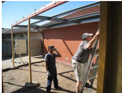
Top: The old roof came down to make way for the new library & interview room
